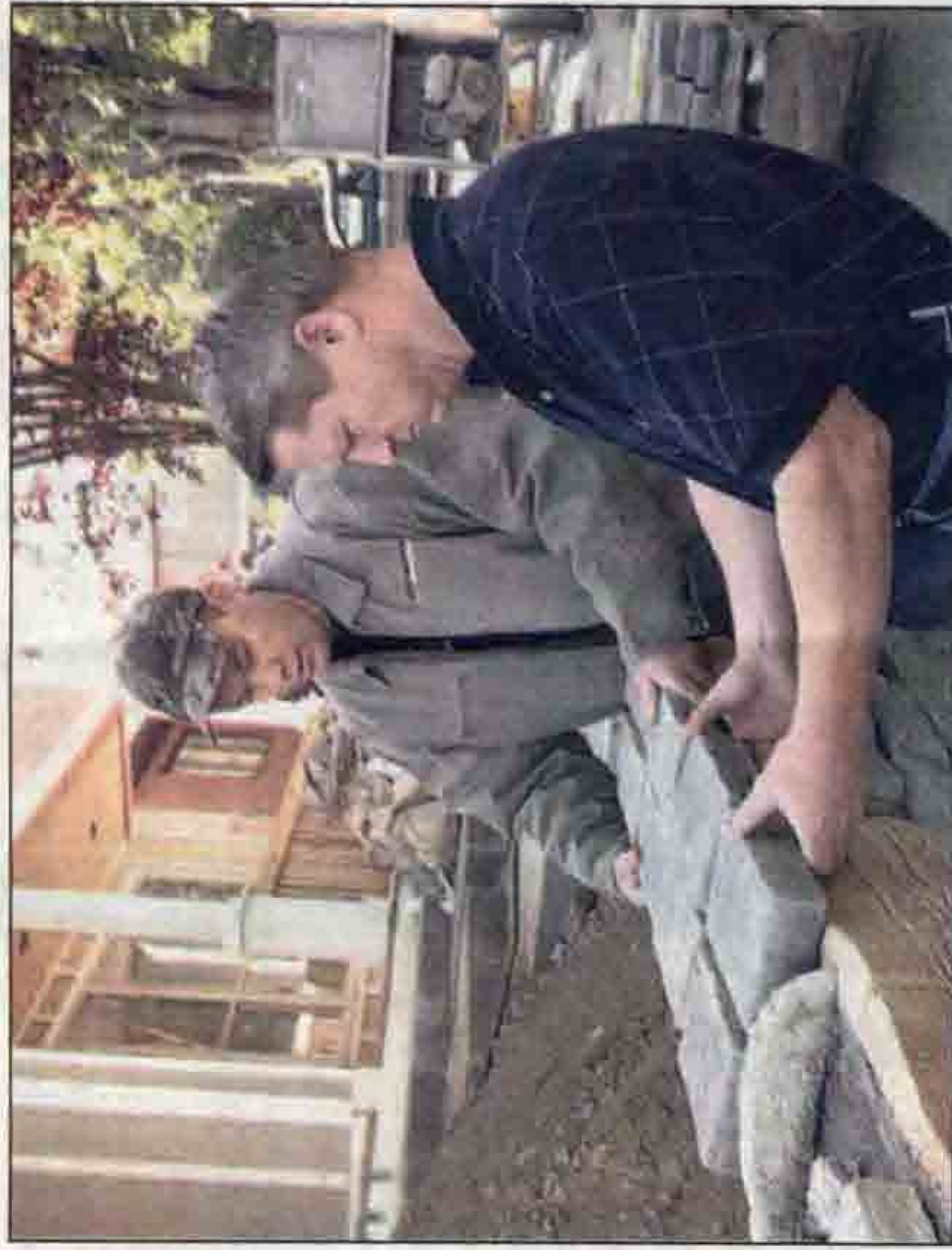
Richard Kassebaum, right, looks over the stone being installed by Pat Bernard of Bernard Masonry in front of a home Kassebaum is building on Southeast 71st Avenue in Portland's Mount Tabor neighborhood. Wanting the home to fit in architecturally with its long-established neighbors, Kassebaum sweated the details such as a classic-looking front door, above left, and an Old Portland-style arch between the living and dining rooms.
